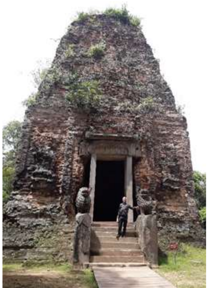
Fig. 2. These structures at Sambor Prei Kuk dating around the seventh century have been supported with supporting beam and concrete pillars (author standing at entrance)
